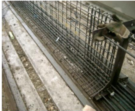
Figure 33: Case PB6. Reinforcement cage and prestressing strands. The picture is taken from (Choulli, 2005).
